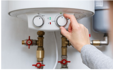
Boilers, furnaces, hot water heaters – combustion gases
